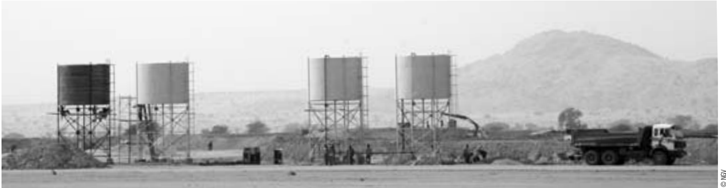
The installations are very basic
